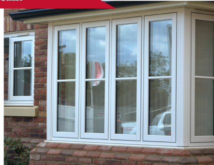
New housing estate - Deceuninck flush sash windows in White Grain and Classic Cream
